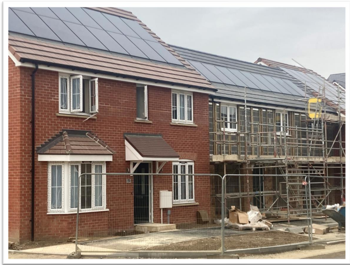
New build with roof solar panels
