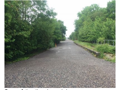
One of the 'haul roads' we are constructing to reduce the amount of construction traffic on local roads.
